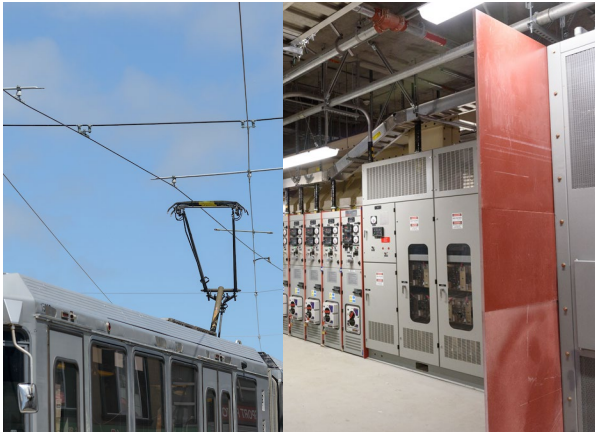
Traction power system
