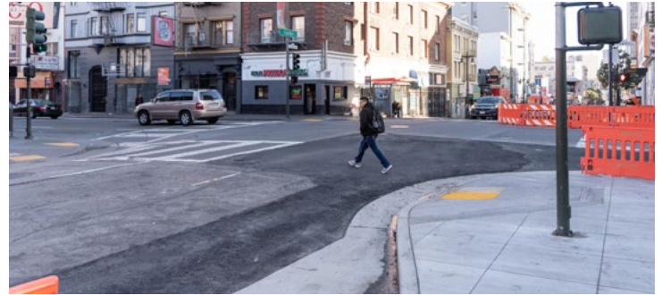
Crews recently installed the first of several pedestrian bulbs planned as part of the project at O’Farrell and Larkin streets.
